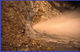
Water burst occurrence during the construction
