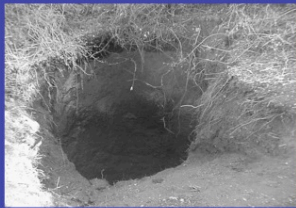
Collapse of the filling of a karstic chimney crossed by Dodoni Tunnel. The collapse outcropped on the surface about 100 m over the tunnel.
